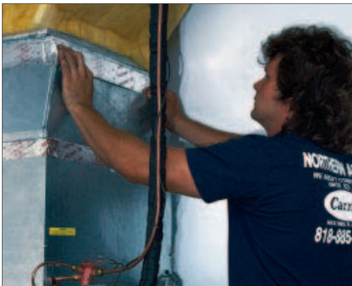
Air leakage and heat loss from ducts add to the load on an air conditioner. Sealing and insulating the ducts allows you to select a smaller unit.
