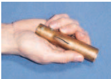
This section of copper pipe split along a weak seam.
