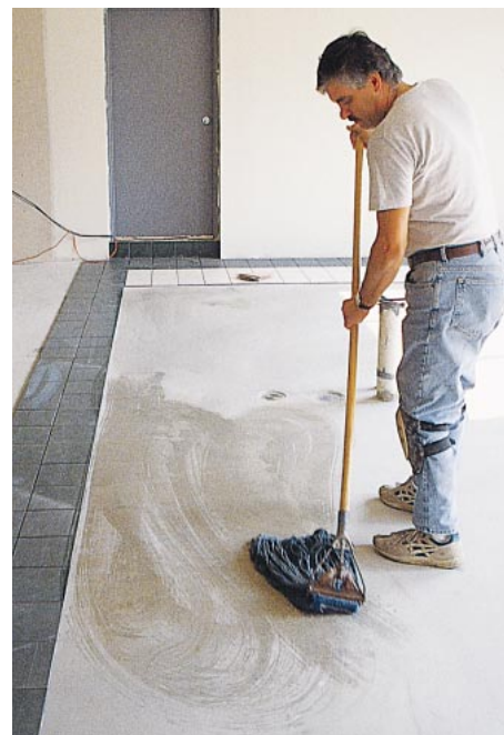
Figure 3. Dirty substrates create poor bonding conditions. Concrete substrates should be wet mopped and plywood substrates damp mopped, with the mop water changed regularly.
