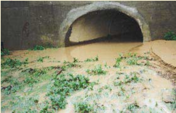
Lack of erosion control at a construction site causes a familiar scene — loose dirt washing into the drain system after a rainstorm.
