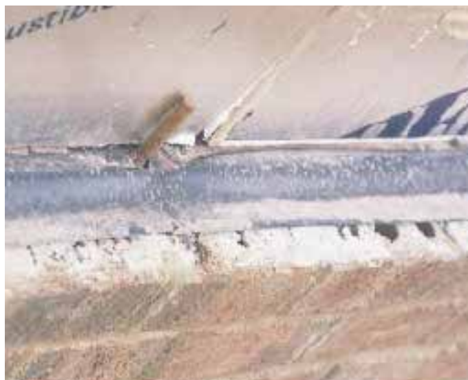
Figure 7. This flashing has been installed incorrectly, since it does not extend all the way to the front face of the brick. Any water is directed into the core holes of the brick instead of to the exterior.
