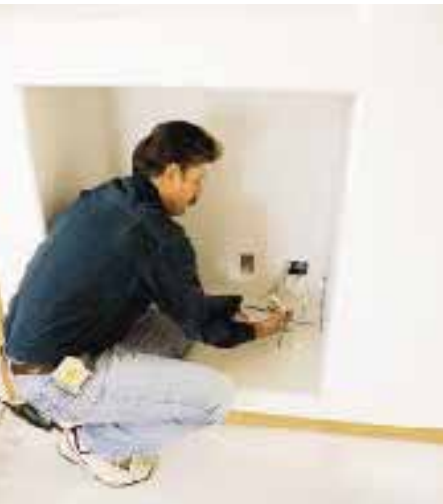
"Standard" house wiring has gone high tech with the inclusion of Category 5 twisted-pair control wiring and RG-6 coaxial cable.
