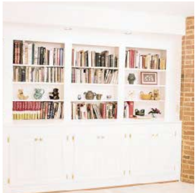
Figure 6. The recessed lighting soffit in front of these built-in shelves looks like it was intended to be there. It actually conceals a beam and ductwork.
