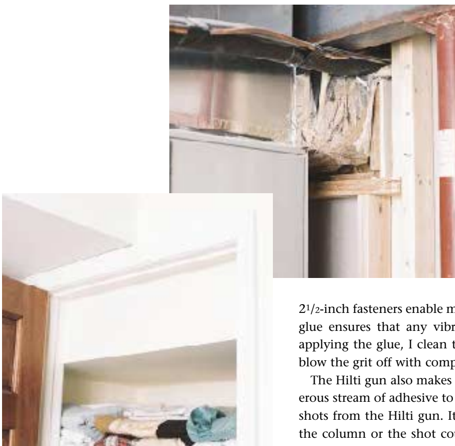
Figure 3. This insulated heating duct (top) was too low to permit adequate headroom, so the author hid it inside a closet. With a full-height closet door (above), no one's the wiser.
