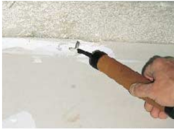
Figure 4. Use a smoke pencil to check the seal between the garage foundation wall and drywall. This joint must be sealed with urethane caulk, an EPDM gasket, or expansive foam to prevent negative pressure from drawing toxic fumes into the basement.
