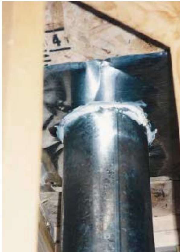
Figure 5. The flue is correctly sealed where it enters the sheet-metal covering at the bottom of the chase. But the edges of the plate should also have been sealed.
