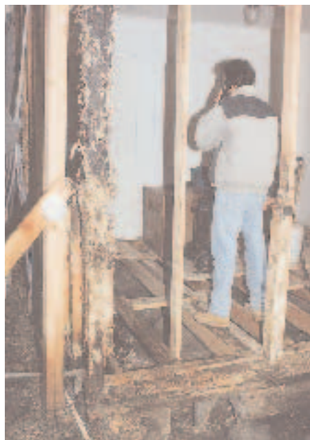
Three months after buying the house, the owner of this house received an unpleasant surprise.
