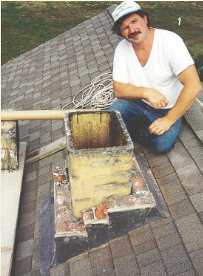
Figure 1. Newly replaced stepped flashing won't stop the leaks in a failed chimney but will remain in place under the pan as a secondary barrier, to prevent wind-driven water penetration.
