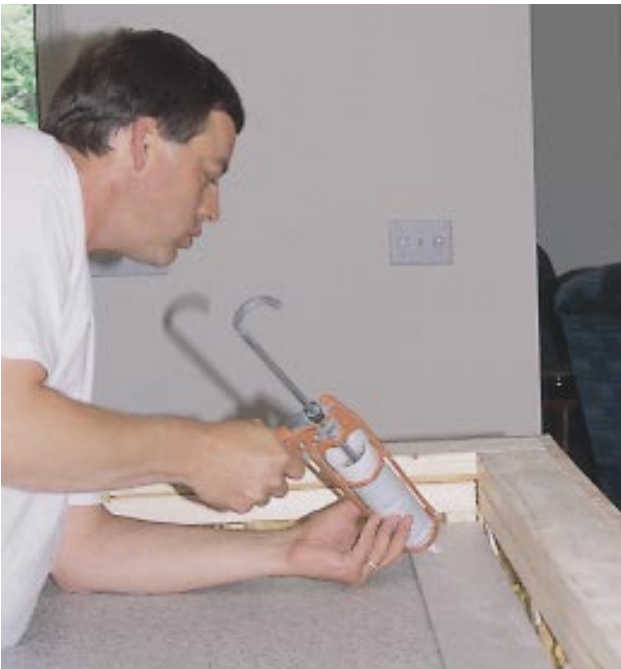
Figure 3. Most solid-surface backsplashes are not attached to the countertop. Such "loose" backsplashes are installed with silicone caulk. Loose backsplashes are much easier to fabricate than coved backsplashes, which are glued to a rabbet at the back of the countertop.
