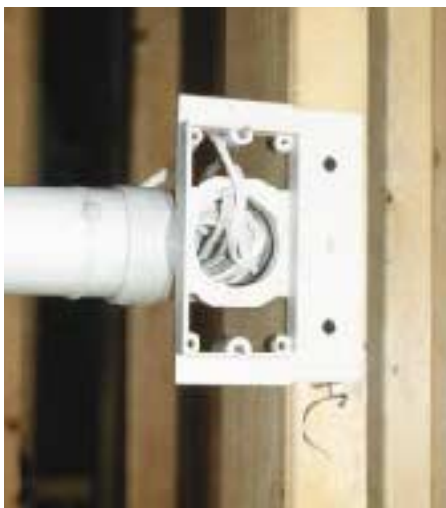
Figure 1. Low-volt, 20-gauge wire makes a home run from each inlet valve to the power unit. Contact points in the hose base connect the circuit to an on-off switch in the wand.
