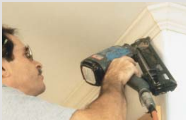
Preassembled corners are easy to install, and the joints are sure to be snug.
