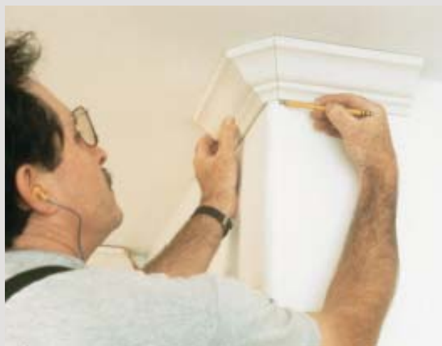
Before any measurements can be taken, bullnose corners must be laid out with a three-piece mockup.
