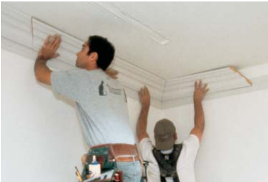
Figure 12. Use a piece of scrap (right), cut with inside-to-inside corners, to ensure proper positioning of the first piece of a corner joint.
