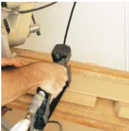
Figure 17. Preassembling splices is faster and guarantees tight field joints. First, fasten the backing to the piece with the inside miter.
