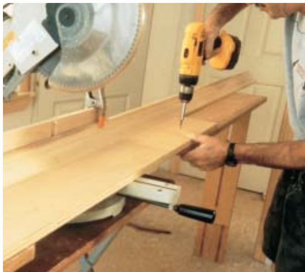
Figure 3. Install a stop along the length of your saw base to stabilize crown molding when cutting in position.
