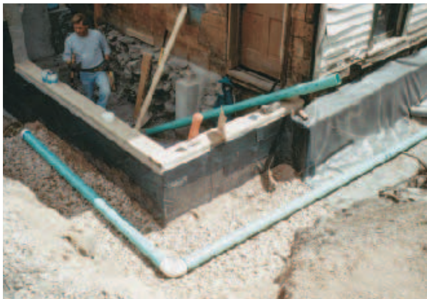
Figure 5. The 40-mil EPDM membrane extends to the top edge of the new shed foundation but overlaps the reinforcing wall, which lies outside the footprint of the building.
