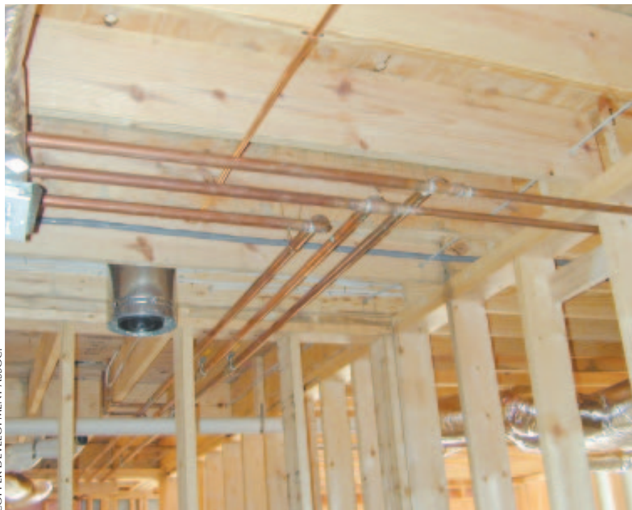
Figure 5. In this home, \frac{3}{4} -inch copper lines tee off from the 1-inch mains on the left.
