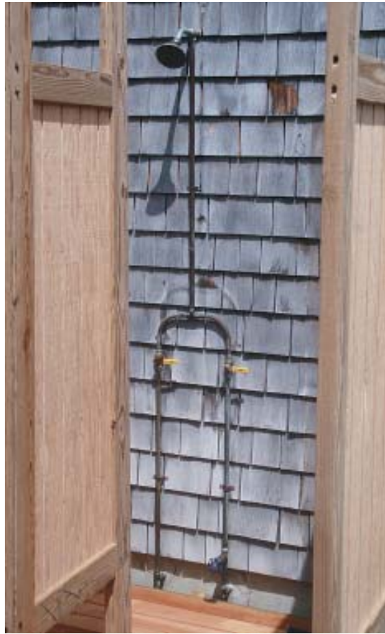
Figure 5. In this shower, the original exposed plumbing, with separate hot and cold stops, was inexpensive, but it was also prone to damage and presented a scald hazard.
