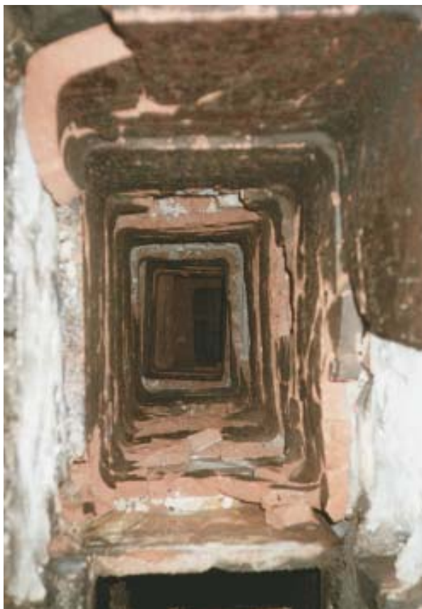
Figure 1. A badly damaged tile flue liner like this one — which shows the effects of repeated chimney fires — leaves the brick and mortar beneath exposed to rain and to the acidic byproducts of combustion.
