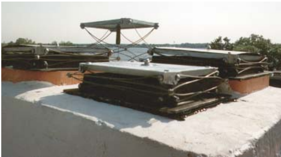
Figure 12. Each flue in the rebuilt chimney top has its own cable-operated damper, which is more efficient and easier to use than a traditional throat-mounted fireplace damper.
