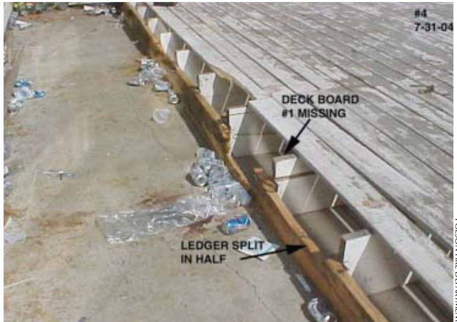
A morning-after photo shows the bottom half of the split ledger board still attached to the otherwise intact deck assembly.
