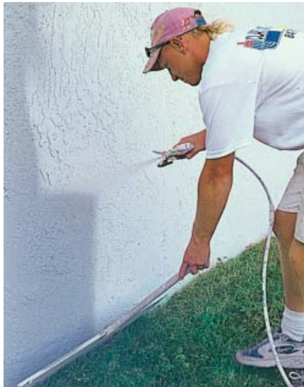
Painted stucco has replaced pigmented applications in some Southwest markets, but suppliers worry that builders aren’t allowing the cladding to cure properly and possibly causing latent moisture problems.
