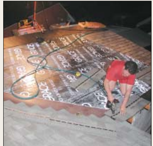
Roofers from as far away as Texas and New York State have traded the slow northern work season for warmer climates and extra-long work hours.
