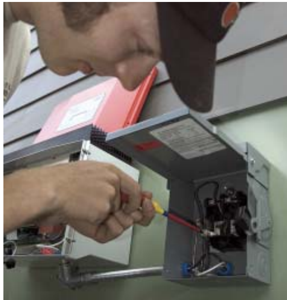
Figure 13. The inverter produces 120-volt AC power, which passes through an AC disconnect on its way to the main service panel. The hole through the lever is for a padlock to lock out the system.
