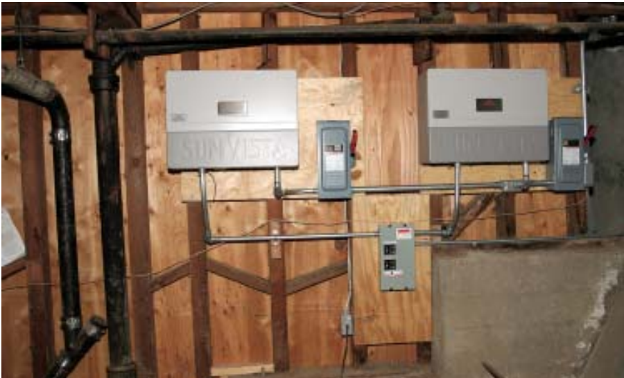
Figure 12. It's sometimes more economical to install two smaller inverters than to go to the next larger size.
