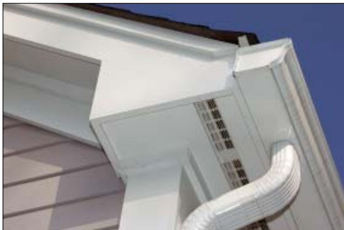
FIGURE 5: Once glued, the many pieces of a PVC cornice fuse together, creating a stiff assembly that remains seamless. These seams are hardly noticeable after three years on a house in Narragansett, R.I.
