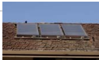
Old solar systems, like the one on this original wood roof, may no longer be operable but can often be put back into service for a reasonable cost.
