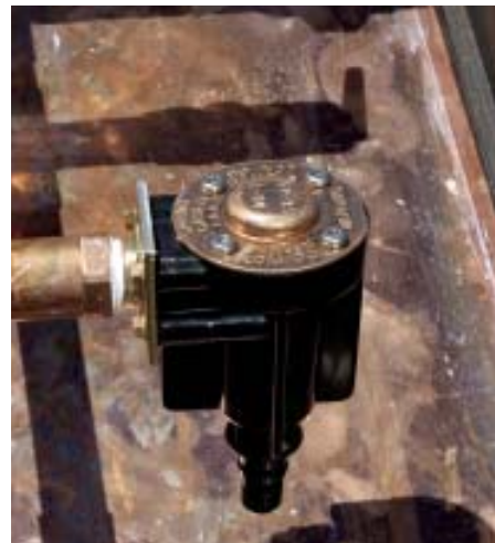
Figure 6. The author's crew always installs a freeze drip valve on the outlet side of the collectors on open-loop systems. If the temperature drops below 35°F, the valve drains enough water from the collectors to bring warm replacement water up from the house.
