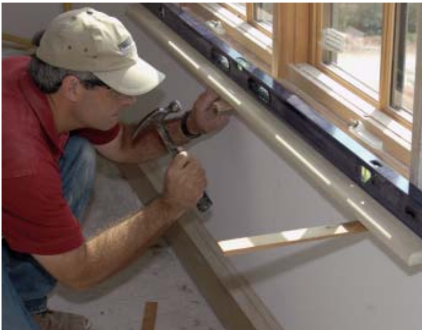
Figure 4. The author uses a level as a straightedge when shimming the stool, which results in an even reveal along the bottom edge of the window.
