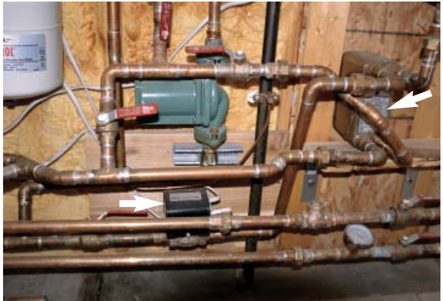
Figure 3. Key components in the author's system include the flat-plate heat exchanger (at right in photo), which heats the domestic hot water loop, and a flow switch (at left), which ensures that the heater fires even at a very low flow rate.
