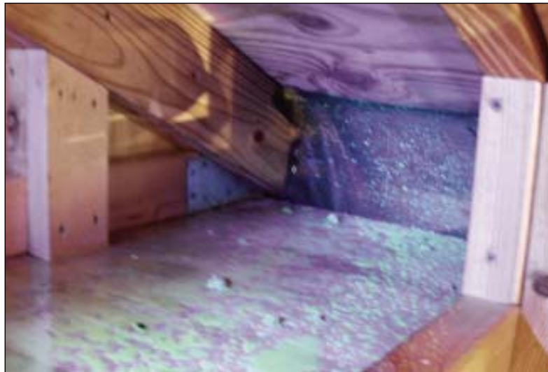
FIGURE 3. Even when soffits are not blown out of place by storm winds, water intrusion can still damage interiors. Here, researchers blew water treated with a fluorescent tracer dye to aid visualization, revealing how water droplets blown by sustained winds through a vented rake along the gable-end wall can accumulate in an attic.
