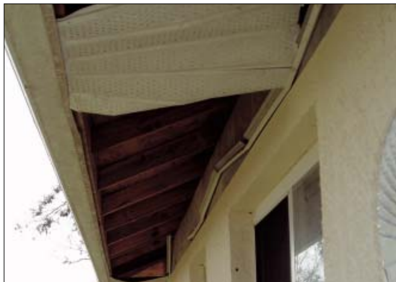
FIGURE 1. Typical soffit attachment details that resulted in blown-out soffits (shown) included securing the soffit with fascia cover or coil stock at the front and using tabbed J-channel against the wall. Tests found that tabbing can work if the tabs are cut 24 inches apart, but that tabs spaced more closely together tend to fail. Even though more fasteners are included with the closer spacing, the integrity of the J-channel is compromised by the repeated cuts.
