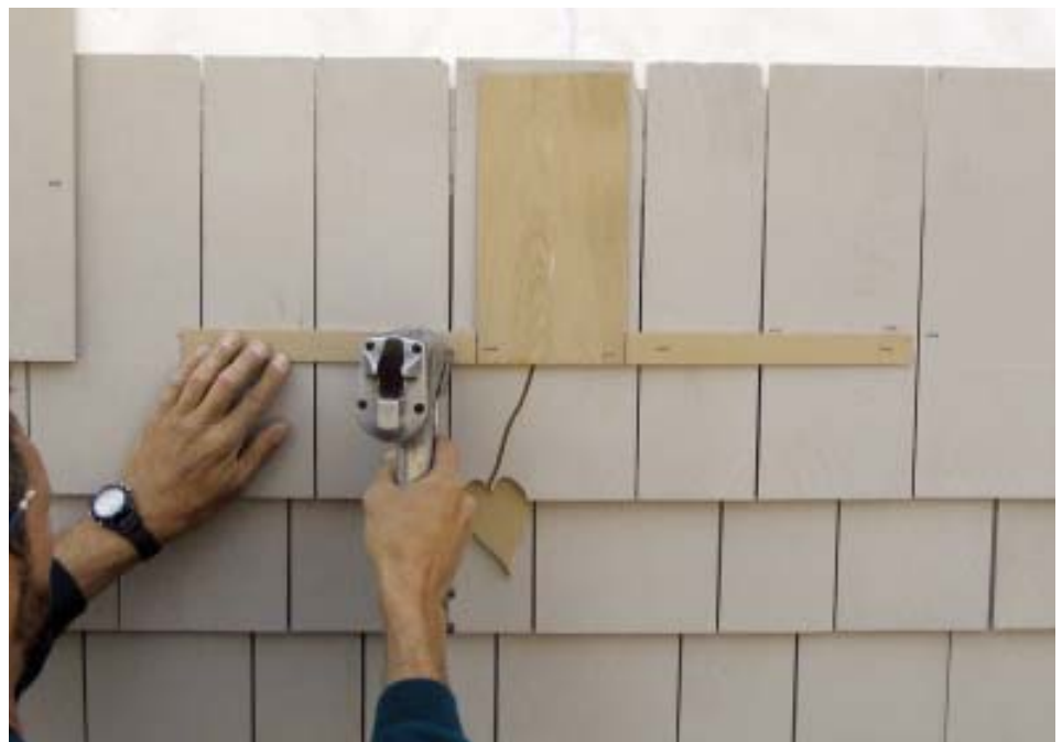
Figure 2. The author installs undercourse shingles at potentially leak-prone spots, then fastens sideways shingle ramps on either side of the undercourse to help transition the overlaying shingles up and over the design.
