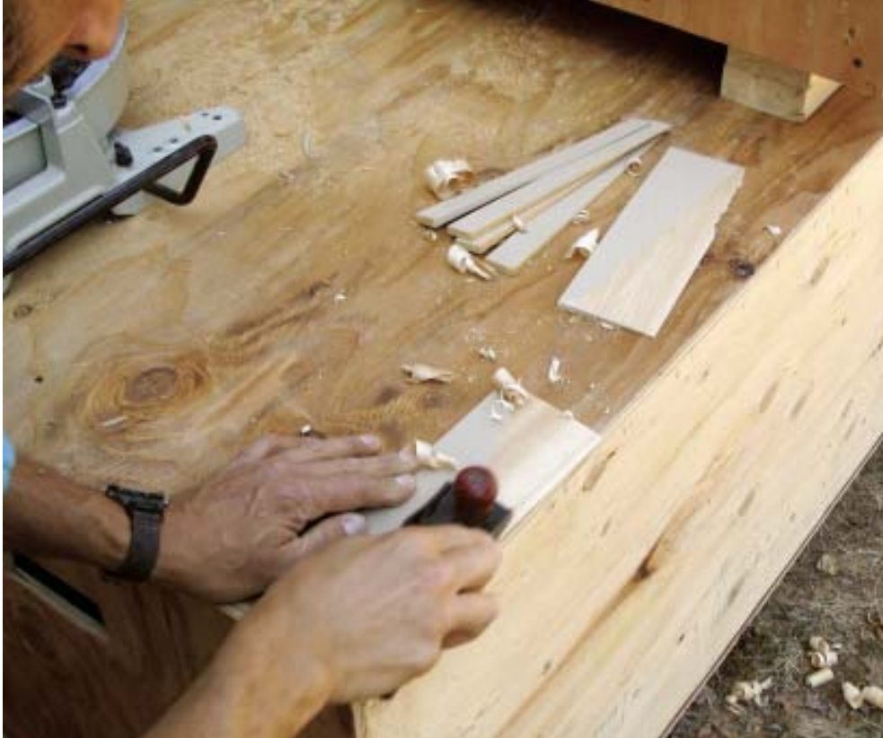
Figure 3. Another way to ease the transition from one level to another when installing decorative shingle patterns is to taper the edge of the shingle with a block plane.
