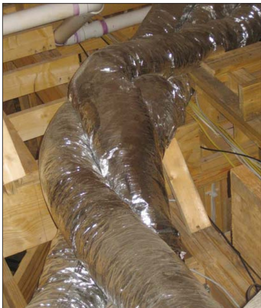
Twisted, tangled flex duct not only slows airflow, but the contact between the ducts cools the contact surface and promotes harmful condensation on the duct surface.
