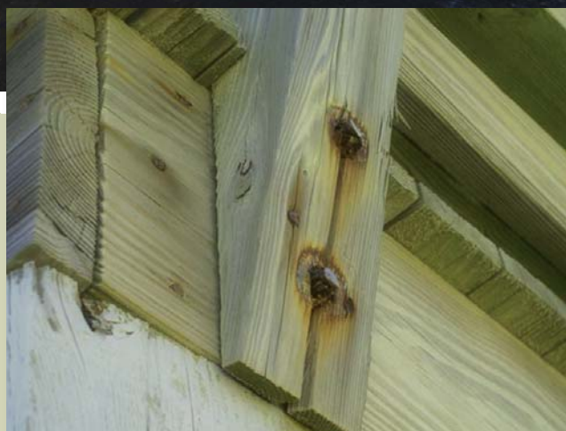
Figure 1. The corrosiveness of the first generation of preservatives to replace CCA took many deck builders by surprise. Lightly galvanized connectors and fasteners, as well as aluminum flashing, often failed in contact with ACQ and CA preservatives.
