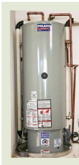
Figure 8. The Polaris (far left) has a stainless steel tank and a simple interface — indicator lights and a dial for setting temperature. This Phoenix heater (left) provides hot-water storage and boiler backup for a solar thermal space-heating (radiant) and domestic hot-water system.
