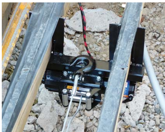
Figure 6. A 12-volt winch powered by an automotive battery operates the lift.
