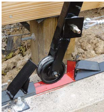
Figure 5. Rollers at the end of the lifting arms travel on tracks made from steel angle. A safety bar placed atop the tracks when the hatch is raised prevents it falling should the cable fail.
