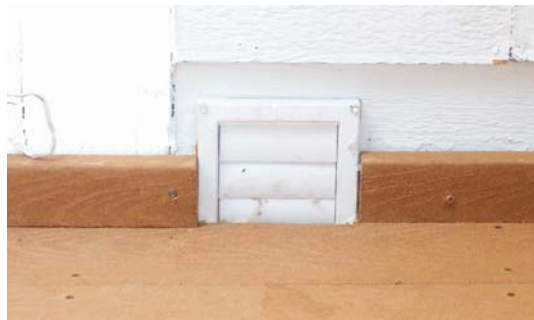
Figure 2. Even a small accumulation of snow would block this termination, preventing the discharge of heat from the dryer and trapping lint.
