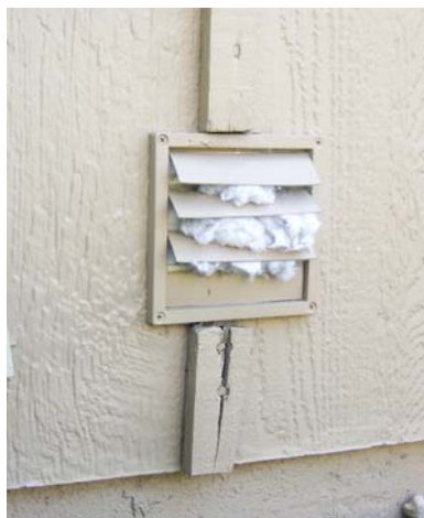
Figure 1. Unbelievable as it may be, this photo wasn't staged. The lint caught in this dryer exhaust termination came through the duct and constitutes a serious fire hazard.
