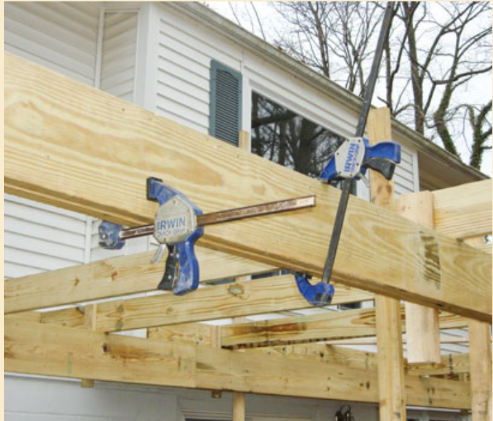
One clamp draws diagonally to align the members of a beam. The second clamp is just snugged in place, ready to be tightened when the beam is lined up.
