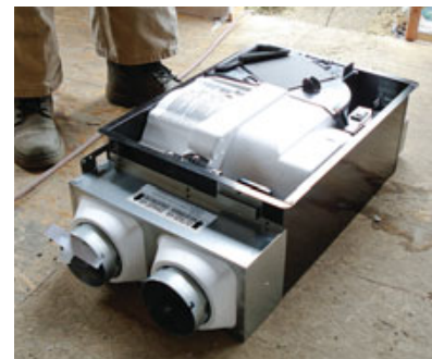
Figure 10. To improve indoor air quality in the now-tight house, the author installed a Panasonic energy-recovery ventilator in the ceiling of the living area. This small, inexpensive unit installs like a bath fan, except that there are two ducts to the exterior instead of one.
