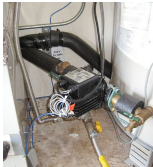
Figure 3. When possible, the author prefers to install the on-demand circulating pump at the water heater in a closed-loop configuration. The pump can be activated by any number of manual switches or motion detectors located near fixtures on the hot-water line.
