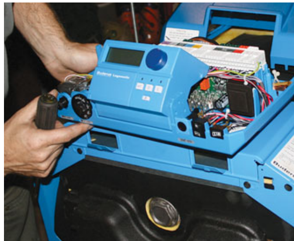
Figure 3. The boiler is controlled by a Logamatic 2107 microprocessor connected to an outdoor air temperature sensor, which modulates the boiler's firing temperature based on demand and weather conditions.
