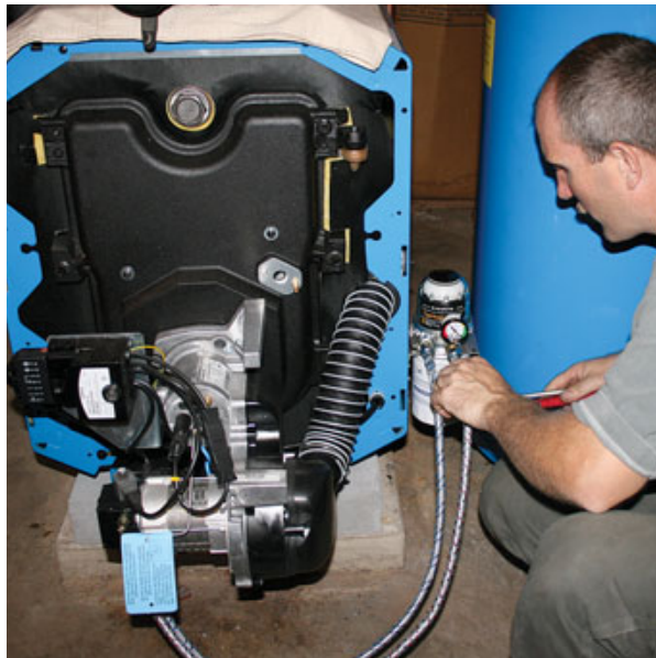
Figure 4. To provide warm, clean fuel for the burner, the boiler is equipped with a fuel line preheater and a 10-micron filter and deaerator, which removes air and gas bubbles in the fuel oil that can interfere with combustion.
