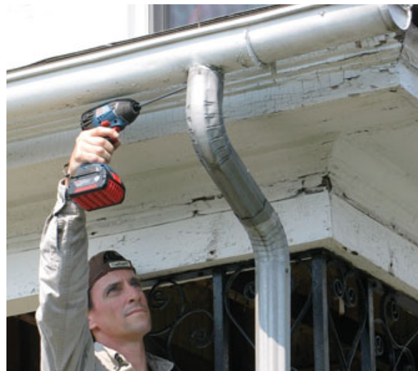
Figure 1. One of the first clues about trouble spots on old porches is peeling paint. Because paint often peels because its substrate is wet, start there when identifying leaks.
