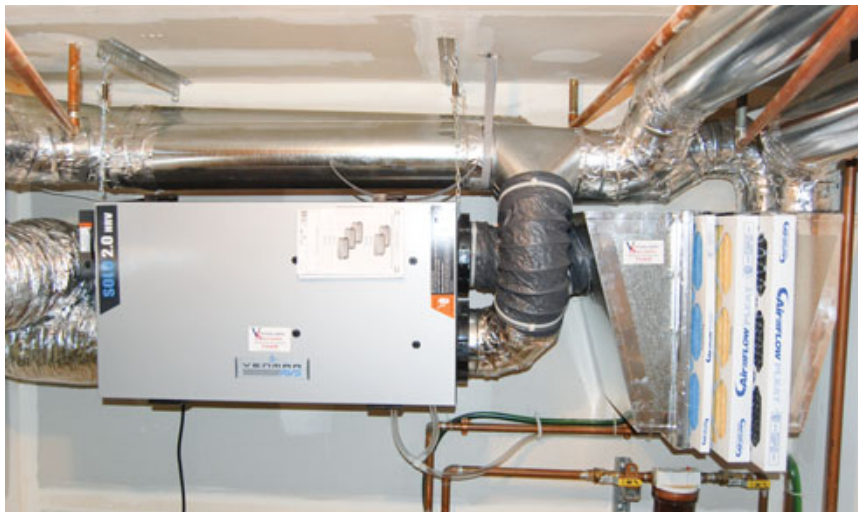
Figure 9. The enclosure to the right of the HRV is a custom-made filtration box with the cover removed to expose the filters. To cut down on noise and vibration, short sections of uninsulated flex duct have been used to connect the HRV to the metal ductwork.
