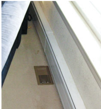
Figure 4. Although supply registers are best placed high in a wall, they can also be successfully installed in the floor. This duct run in a joist cavity (far left) terminates at a boot that supplies a floor register (left). Convection currents from the heat strip will help to mix the incoming air with the air in the room.
