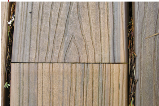
In this Washington state deck, the ends of the capstock decking have swollen after installation.
