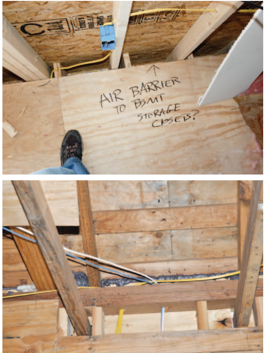
Figure 3. The gap between the subfloor and wall sheathing in this home (top) allowed unconditioned air to flow through a basement closet equipped with an outside door and into the living space above it. Smaller gaps between the framing and sheathing at the eaves — and around pipe and wire penetrations in partitions — were sealed with black canned foam (above).
