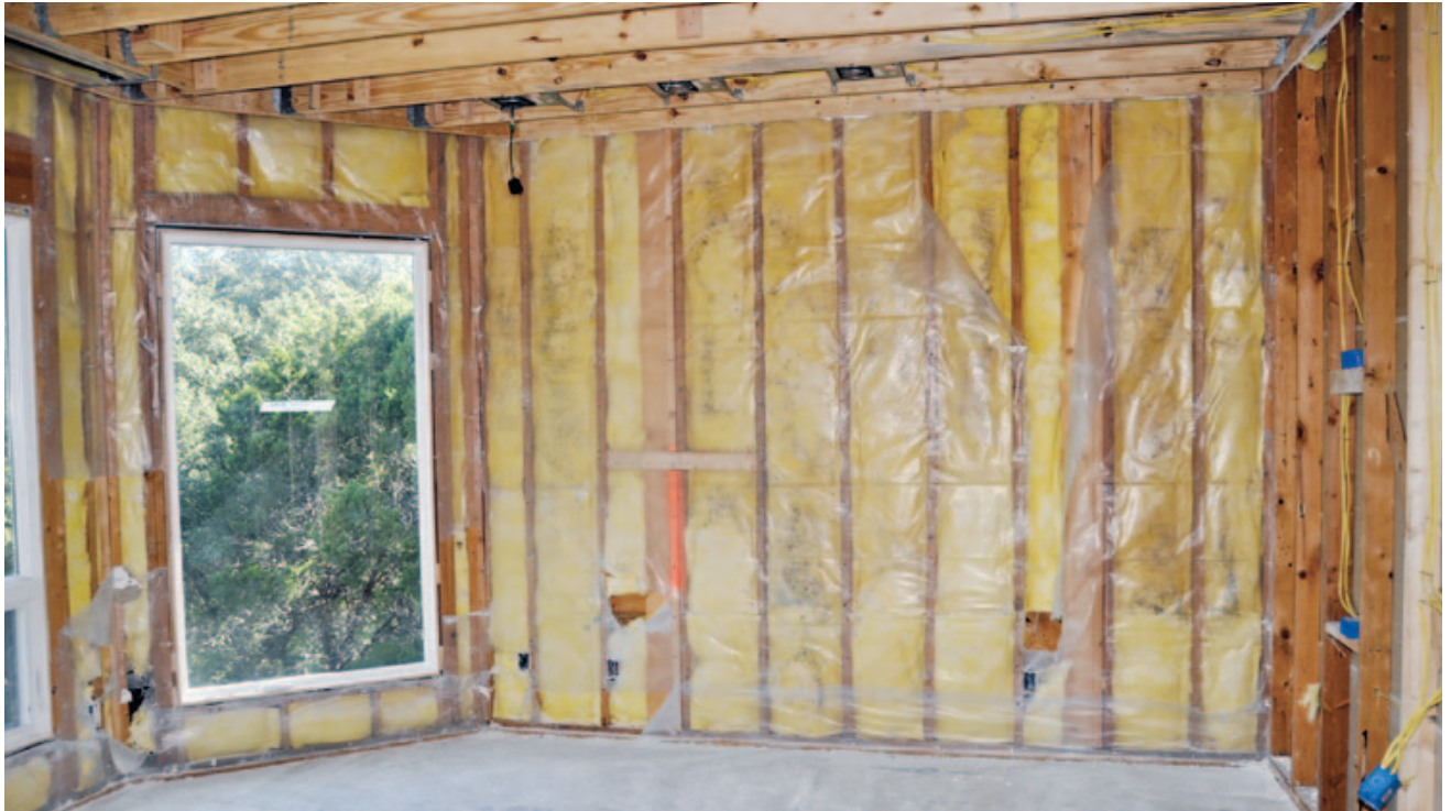
Figure 1. Water vapor from humid outdoor air has condensed on the cold surface of the interior poly in this 10-year-old home, creating a zone of chronic dampness. Note the black patches of mold on the fiberglass batts.
