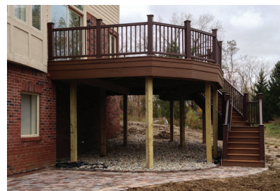
Although these 6x6 PT posts are structurally sound, they look under-sized and unfinished.
