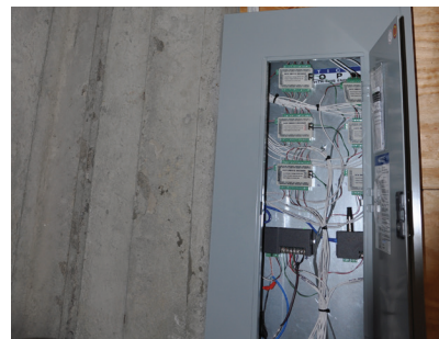
The circuit for each rail segment is wired to a panel in the basement.
