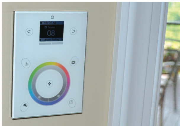
The basement panel is connected to a touch-screen DMX controller mounted in the living room.
