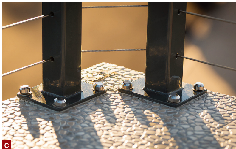
Figure 3. Besides being undersized, the original, single-corner posts required a sharp bend in the cable, which prevented proper tensioning (A). The author prefers double corner posts, which offer a more gradual bend for the cable and a more secure corner attachment for the ipe top rail (B). The posts are equidistant and located a minimum of 4 inches from their centers to the corner, which creates a soft, 45-degree cable bend at each post (C).
