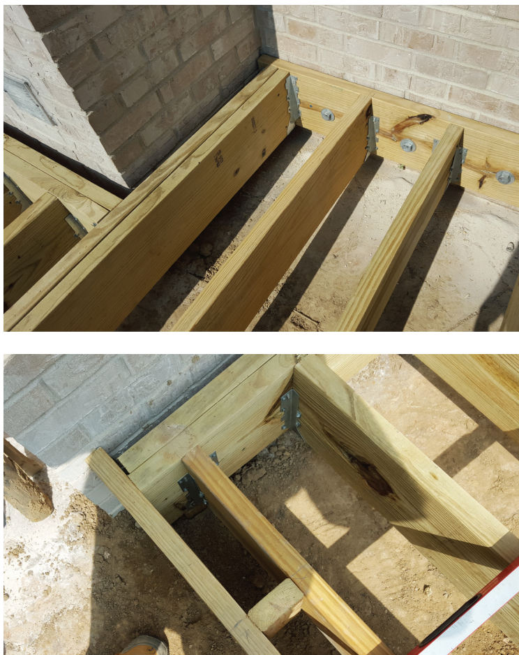
Figure 4. The ledger couldn't be attached to the masonry chimney, which requires a 1-inch minimum gap between the brick and the framing (top). To support the framing at the corner of the deck near the chimney, the author had to install a post, which extends about 9 feet below grade and bears on the chimney footing (above).
