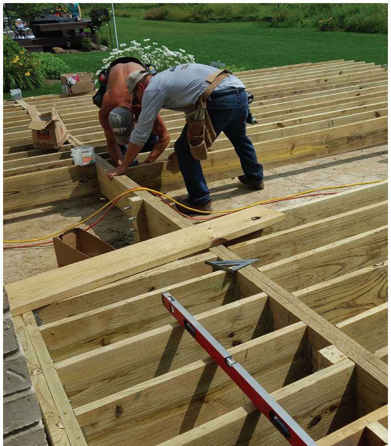
Figure 6. Because the composite decking would be installed at a 45-degree angle to the framing, the joists were installed on 12-inch centers to meet the decking's span requirements.
