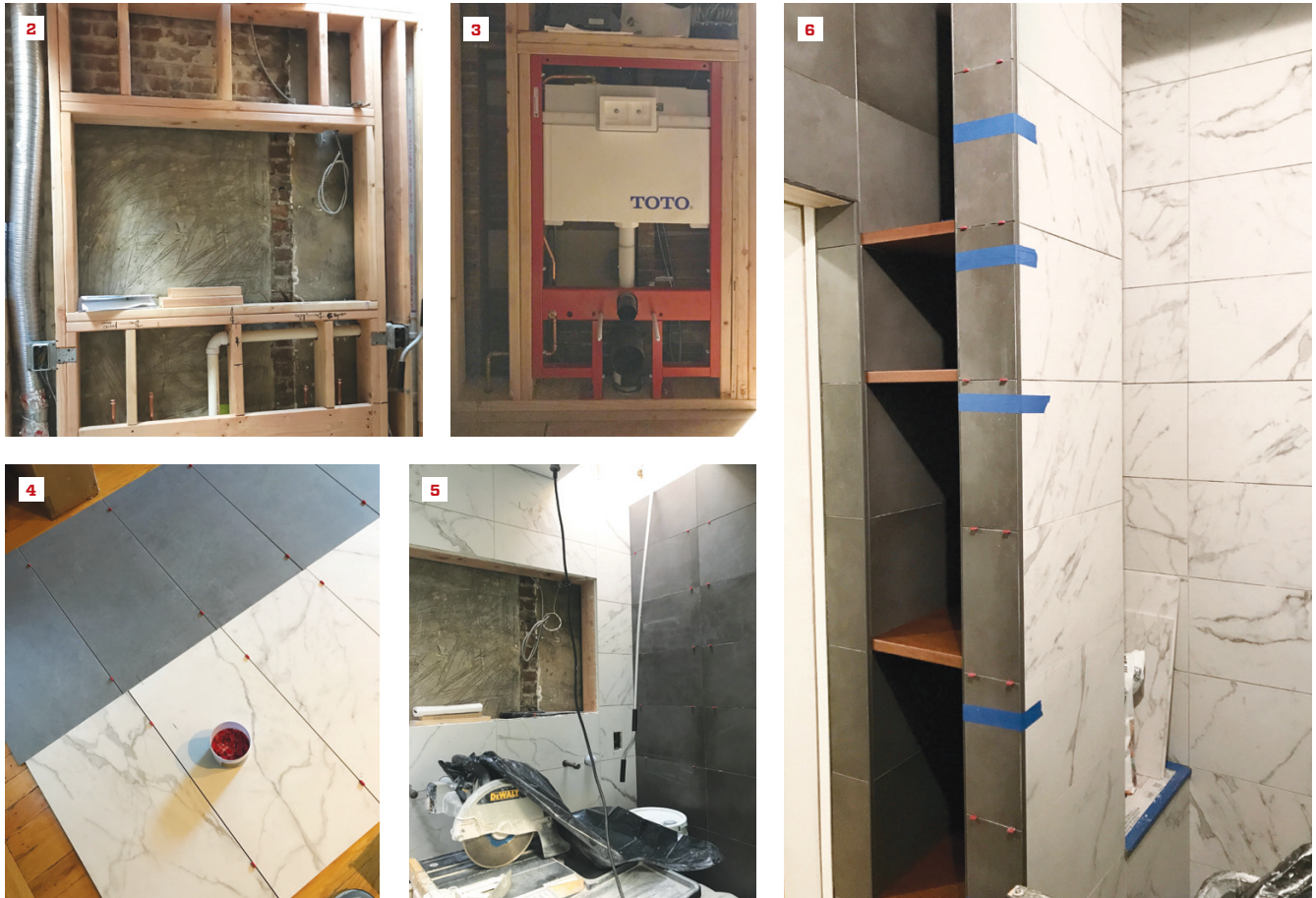
New 2x6 wall framing and solid blocking were needed for the wall-hung vanity and recessed cabinet above (2) and for the toilet's in-wall tank and mounting system (3). The two wall-tile selections were slightly different sizes (4), requiring different-sized grout joints to ensure that they lined up in the corners where they met (5, 6).
